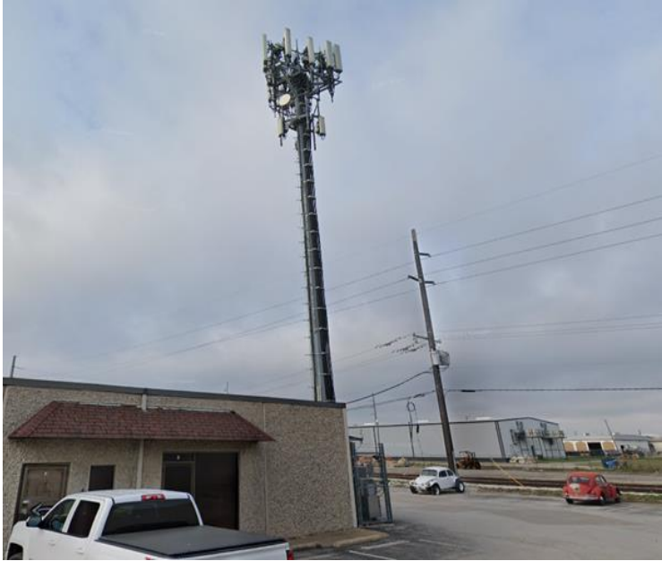
Existing Cell Tower on the subject site.
