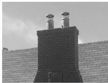
Exposed pre-finished chimney terminations are inappropriate.
