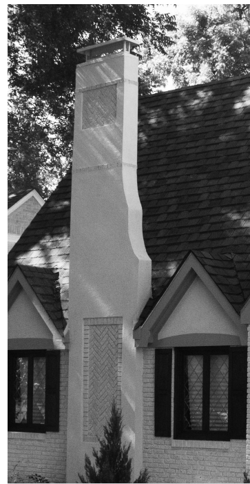
Chimney depth does not reflect traditional masonry construction.
