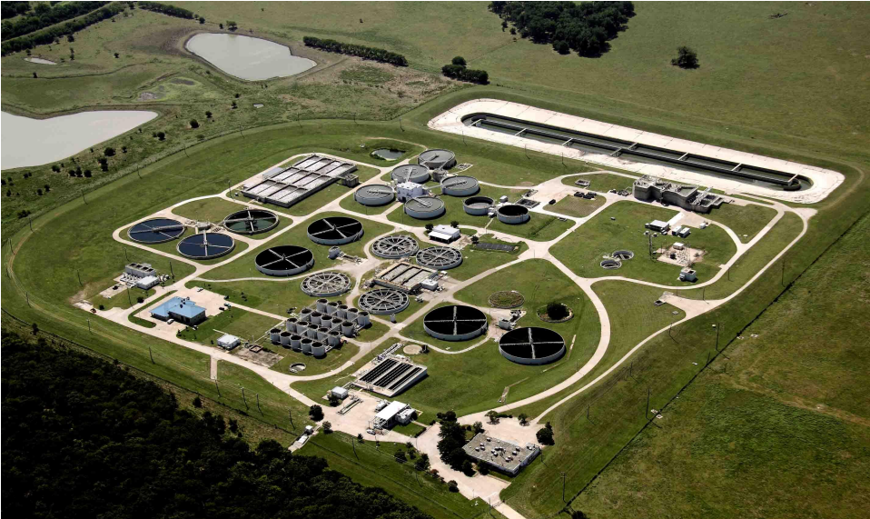
Duck Creek WWTP (Sunnyvale, TX) Treats 40 MGD.
