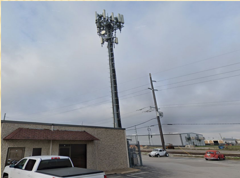
Existing Cell Tower on subject site.
