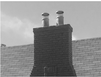
Exposed pre-finished chimney terminations are inappropriate.
