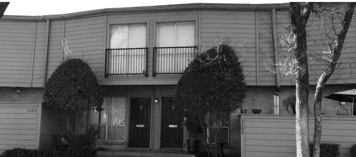
Balcony has no base making it unusable and inappropriate.
